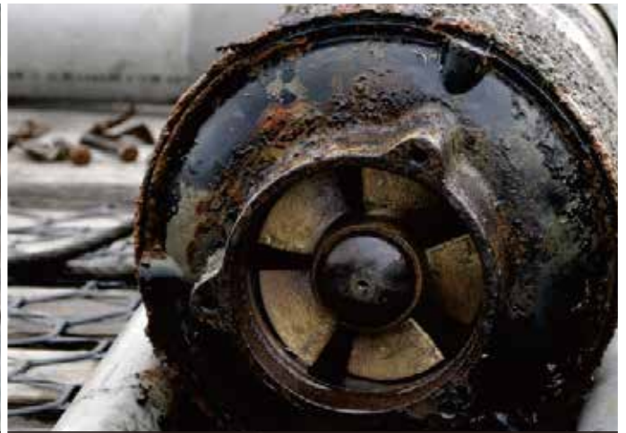
With sacrificial anode : 5 months pumping in seawater applications
